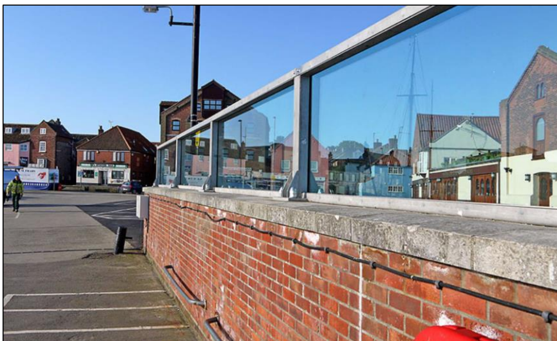
Plate 4.5 Example of a glass flood barrier installed along a wall
